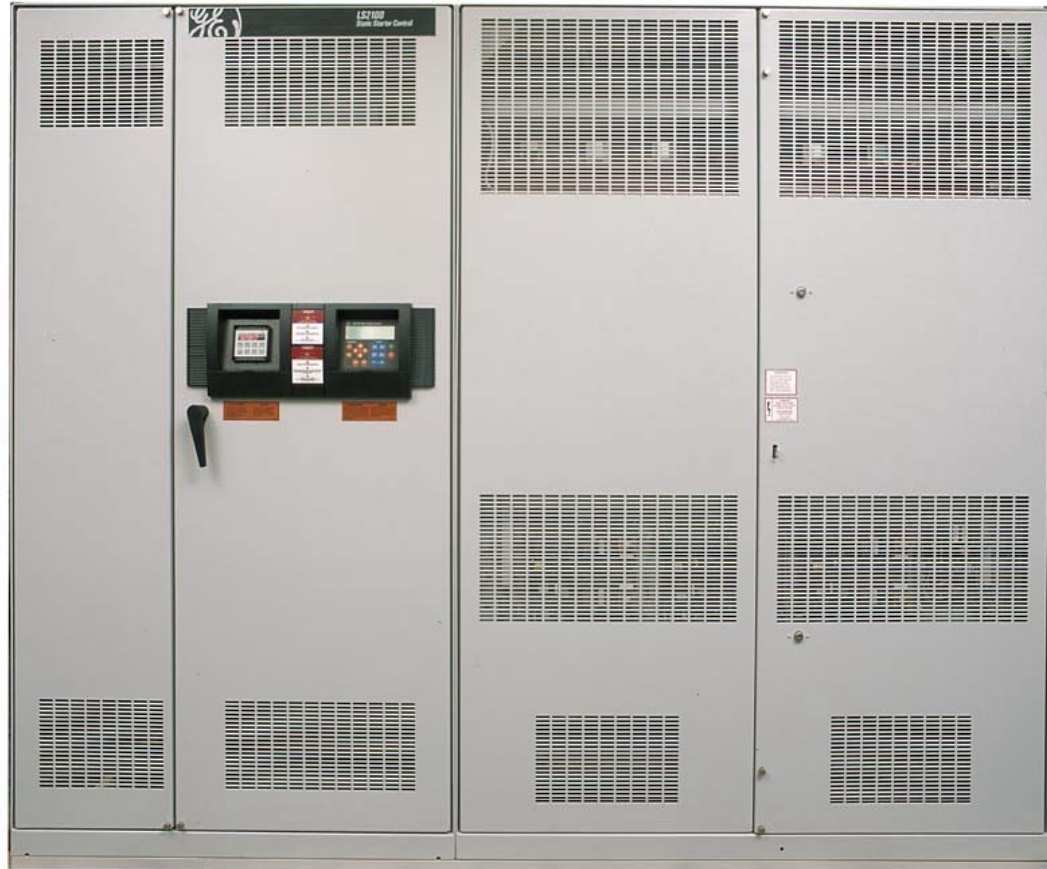
MVA Static Starter Enclosure
